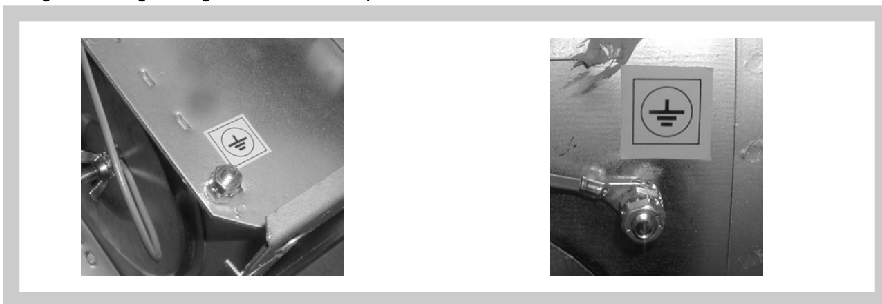
Fig. 4 The grounding screw on the fire damper
