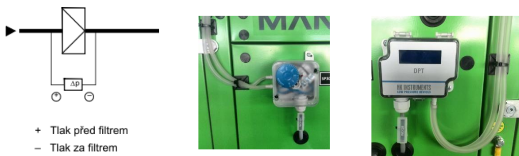
Figure 12 – Wiring of manostat inlets and installation on the shell of the air-conditioning
